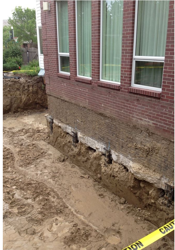
This photo shows the ECP PPB-300 Steel Piers™ installed on the structure and the piers have been
