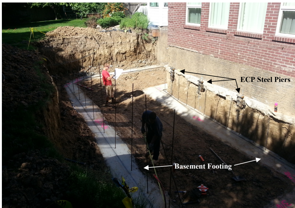
The steel piers have been installed, the excavation is complete and the new basement footings are in place ready for the new basement walls.
