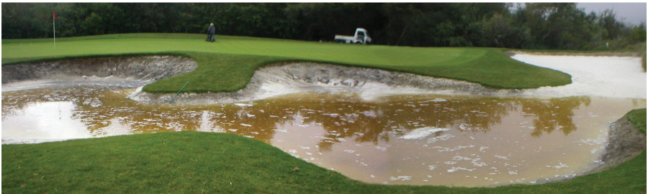
Before: Flooded Sand Trap
