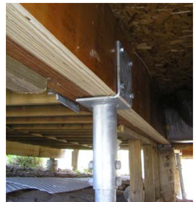
The photographs above show the pile installations in the tight conditions under the structure.
